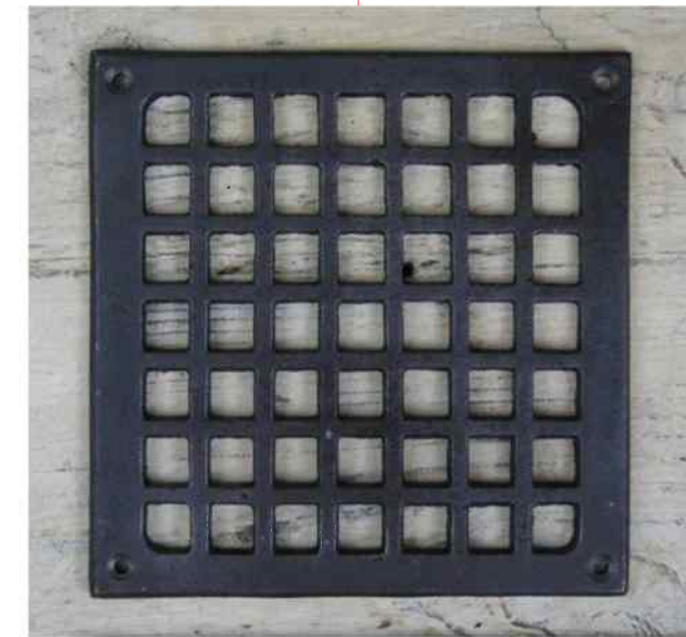
Cast Iron ventilation grille with fly mesh at external termination
